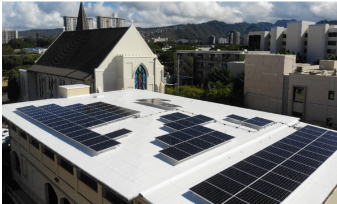
The 88 solar panels on the Parish Hall roof
